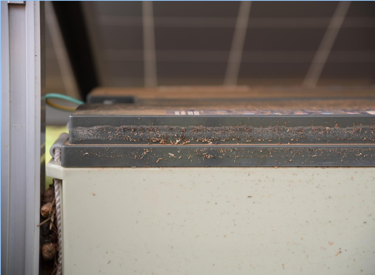
Jan 2018: Tile F8's batteries had been completely submerged. The height of these batteries is 240mm, indicating a flood level of at least 220mm.
