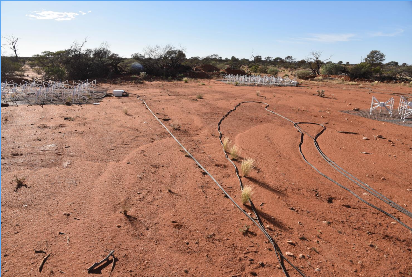
April 2017: Land cleared for installing a dense array of MWA Tiles causes changes to the direction water flows and the locations that the water pools. The result of this caused damage to the equipment in the newly formed flood plain.
