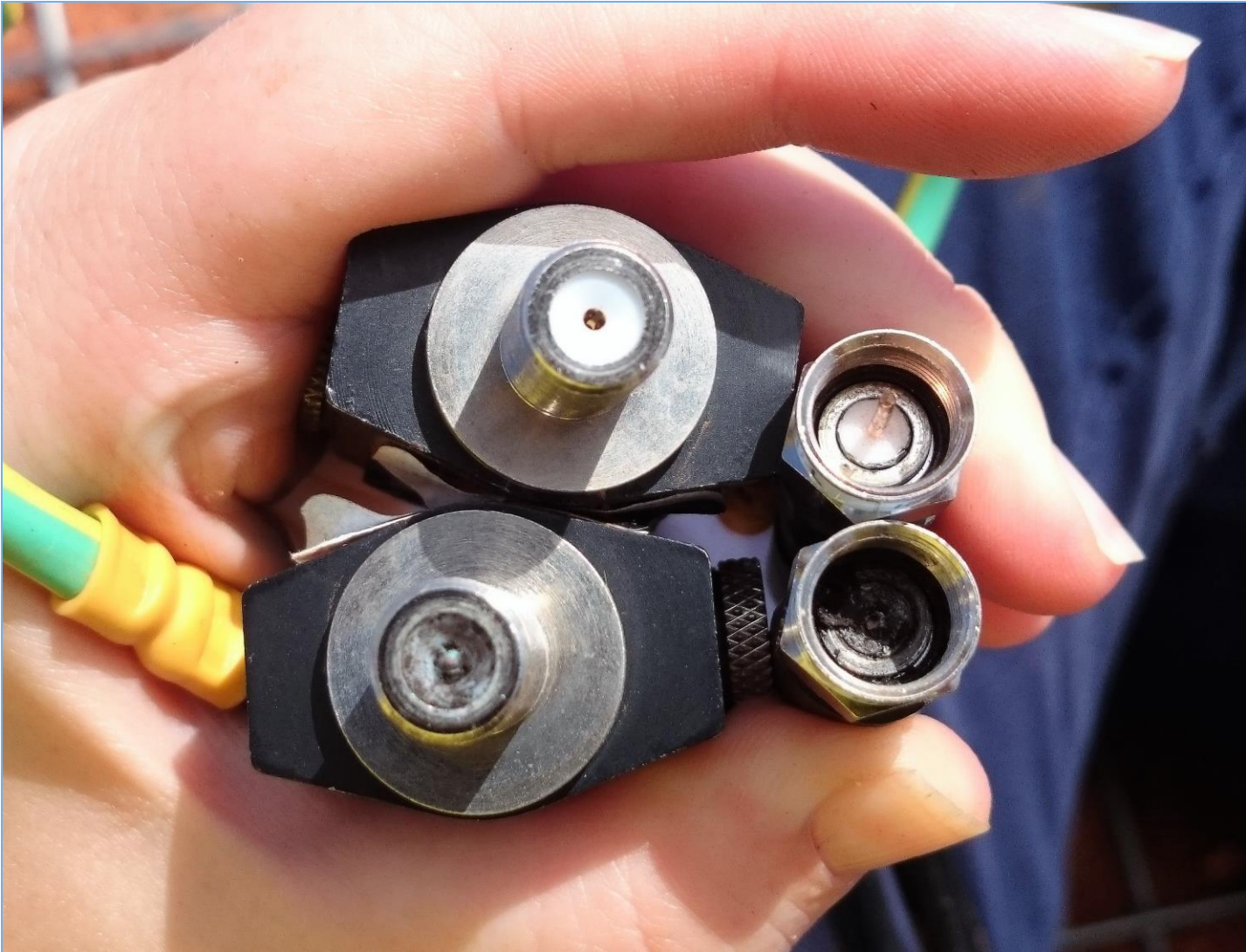
April 2017: Submerged cables exhibited signs of damage at the lightning arrester connectors due to a combination of water ingress and current transmission.
