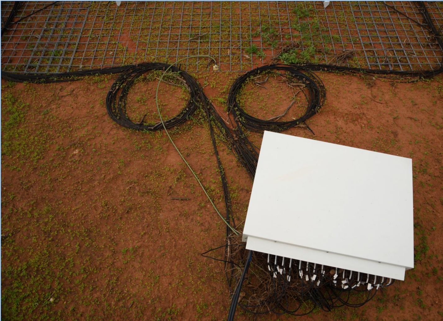
Jan 2018: Tile F8's beamformer had been physically shifted by the water flow.
