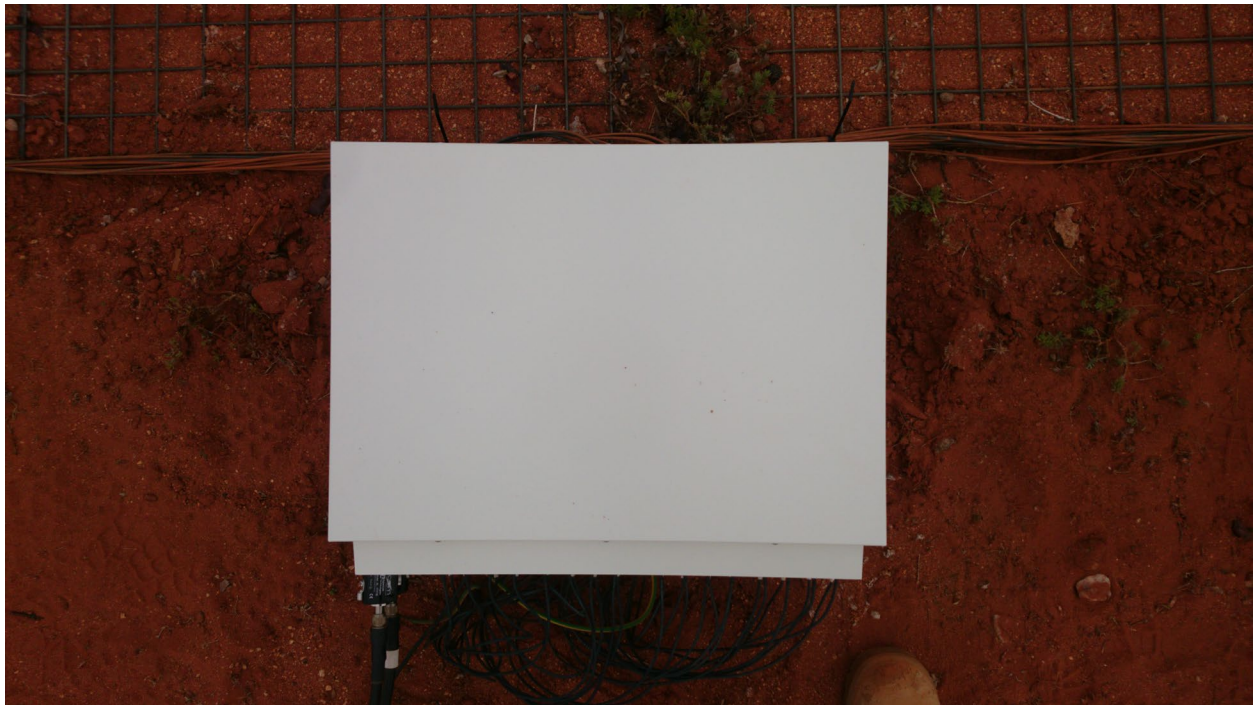
FIGURE 1: TOP VIEW OF NEW STYLE LNA CABLE MANAGEMENT
