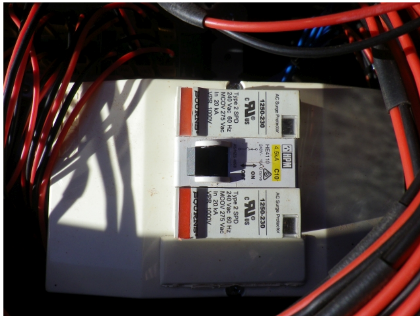
FIGURE 4: APIU INTERNAL SUB-BOARD SHOWING BREAKER AND SURGE PROTECTORS
