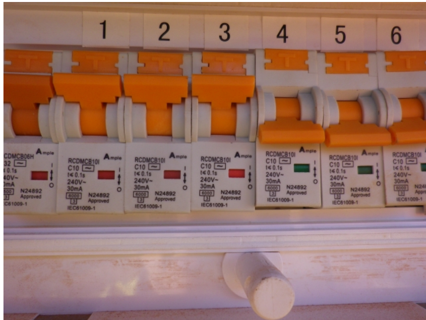
FIGURE 3: AAVS1 POWER DISTRIBUTION SUB-BOARD BREAKER PANEL SHOWING BREAKER "3"
