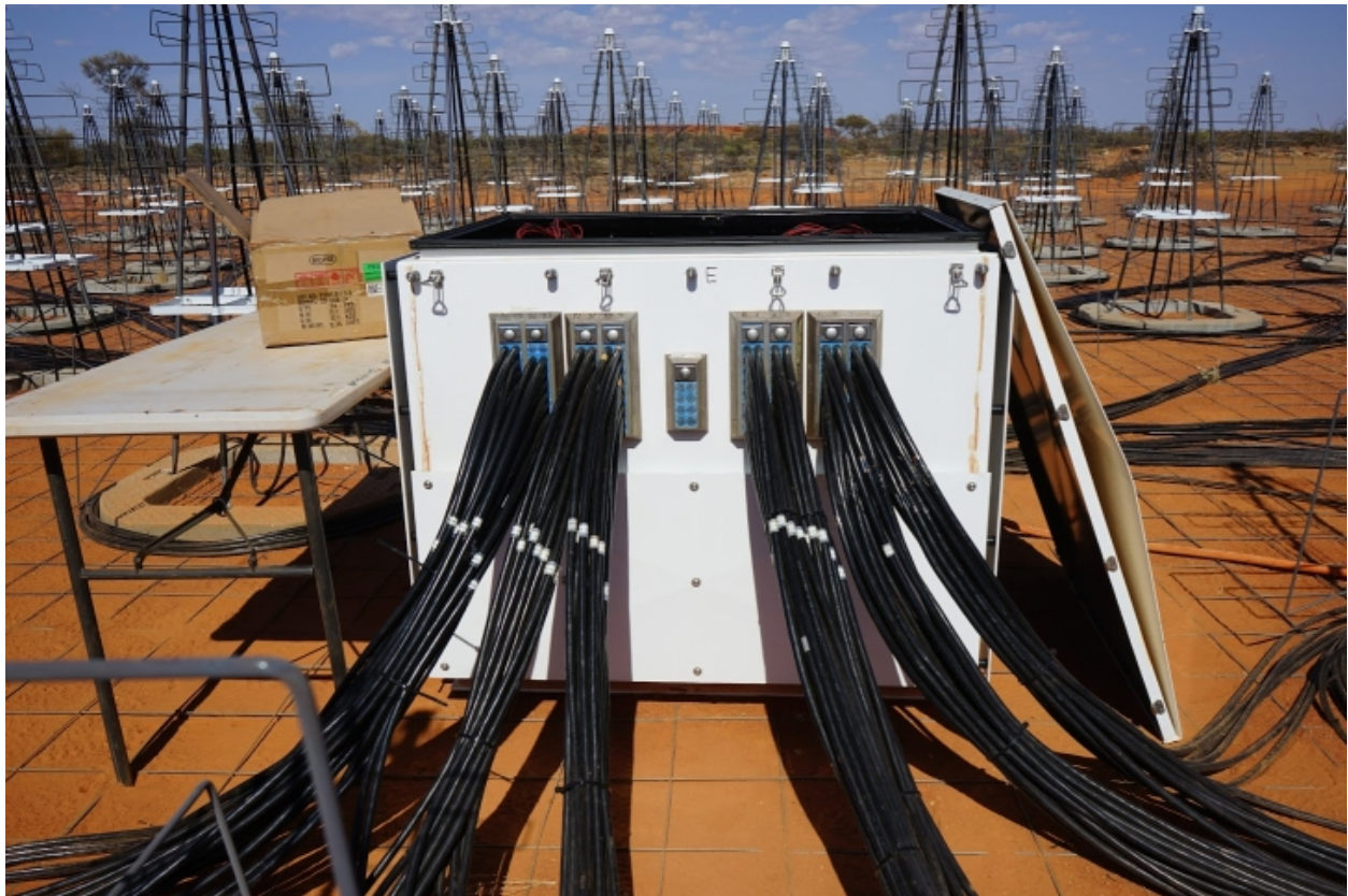
FIGURE 1: NORTH FACE OF APIU ON AAVS1.1 ANTENNA ARRAY
